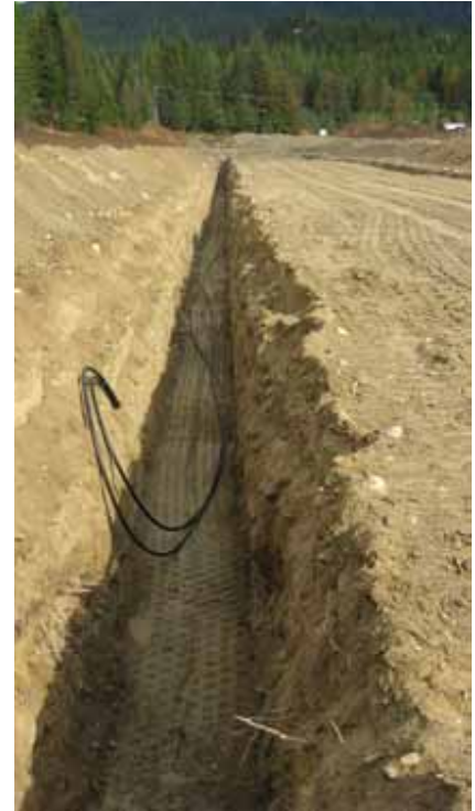
The trench for Crawford Bay School's geothermal cables bisects the playing field
